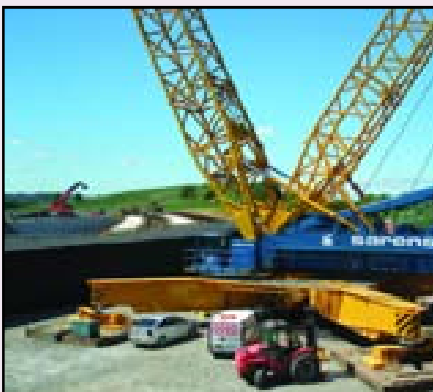
Construction work at the M74 extension in Glasgow – ScotAsh provided material for bridge abutments
