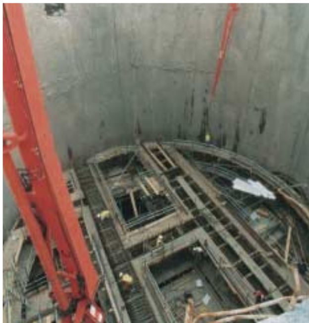
The Ayr Pumping Station. Photo courtesy of West of Scotland Water
