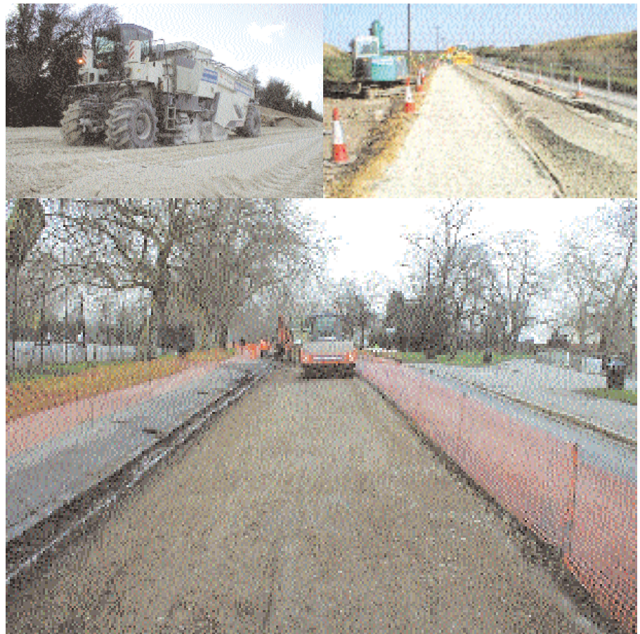
Work under way at Finsbury Park (main picture) and the remediation project at Rainham Landfill site, above.
