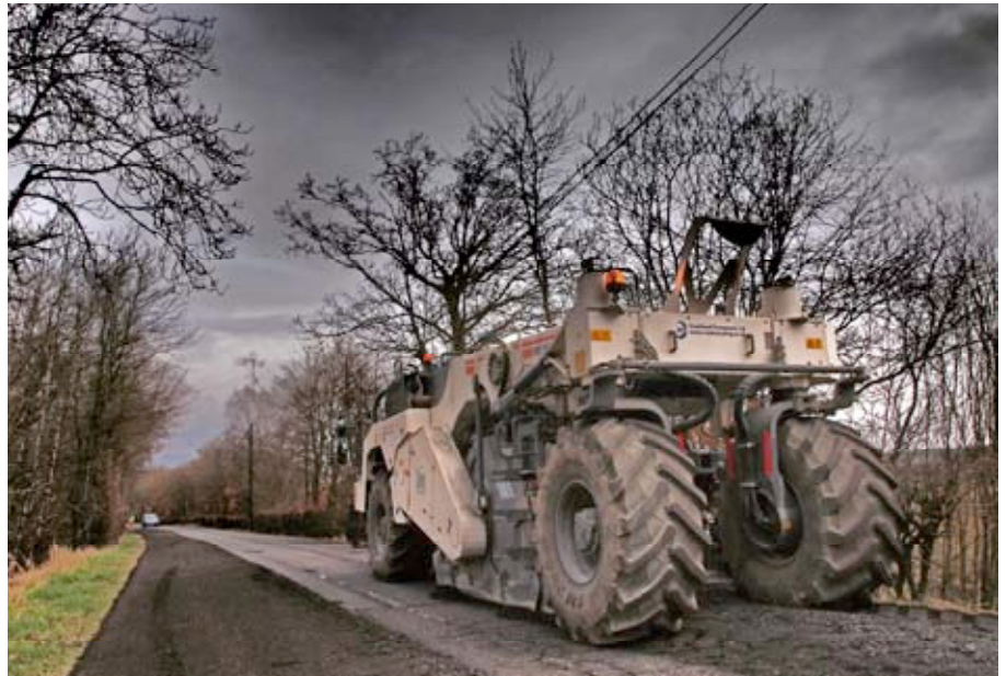
Rip it up and start again: The Wirtgen 2000 road recycler pulverises the pitted and worn road surface
